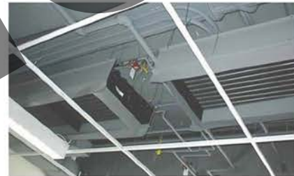
7. ACTIVE CHILLED BEAMS
