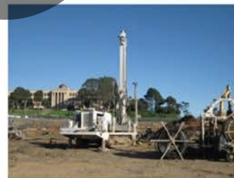
3. GROUND SOURCE HEAT PUMP
