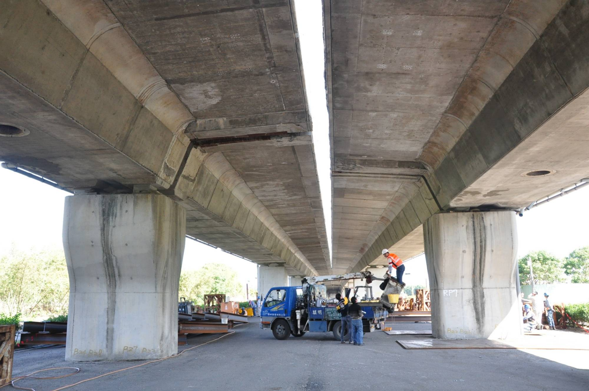
Gap between two bounds @ Exp. Joint
