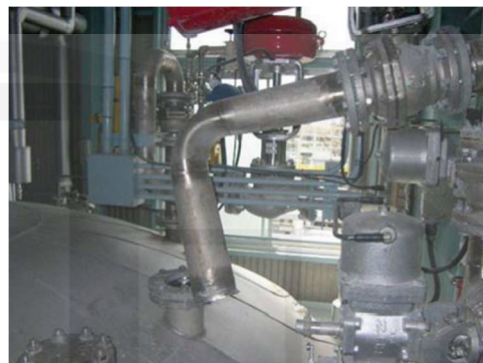
Fig. 1. Seismic damage to hydrogen pipelines in a petrochemical facility (Wada et al., 2013).
