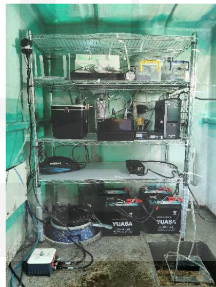
Fig. 4. Interior layout of the monitoring station in the Gengziping area
