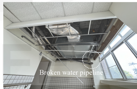
Fig. 2. Failure of the air handling unit
