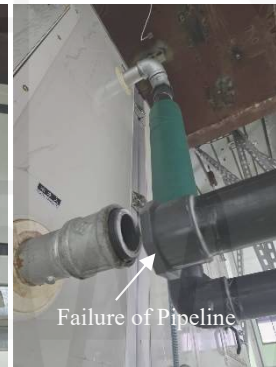
Fig.9. Failure of pipeline
