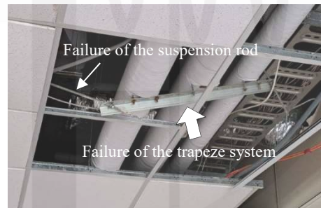
Fig. 1. Failure of the trapeze system
