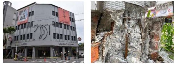
(a) Exterior of the building (b) Cracking of concrete at the base of the column
