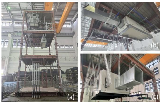
Fig. 4. (a) Pipeline system on the first floor; (b) Air handling unit on the second floor; (c) Air handling unit on the third floor
