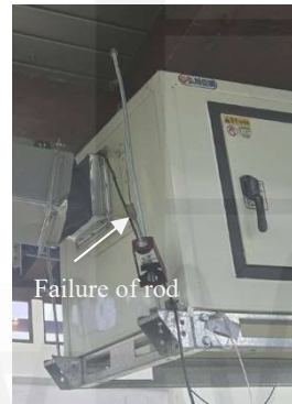
Fig.8. Failure of rod
