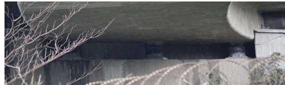
(a) A2橋台側向止震塊開裂
